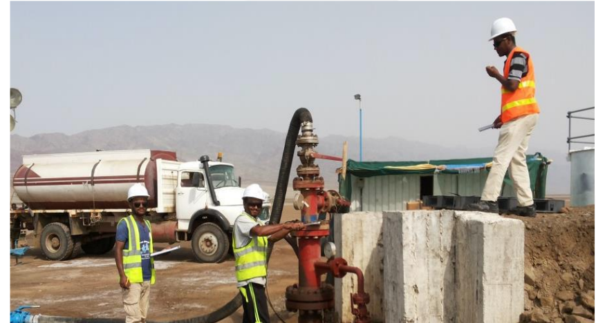
Solution Mining Well Head
